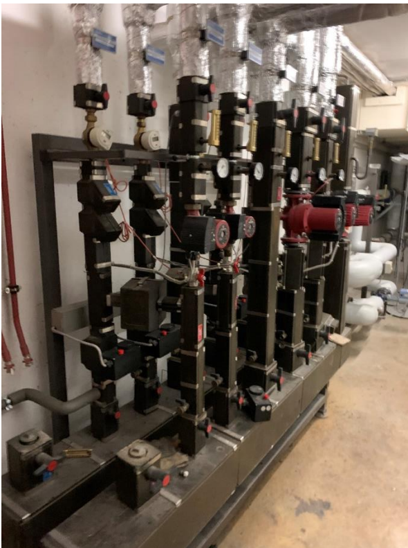
Heat distribution, district heating
